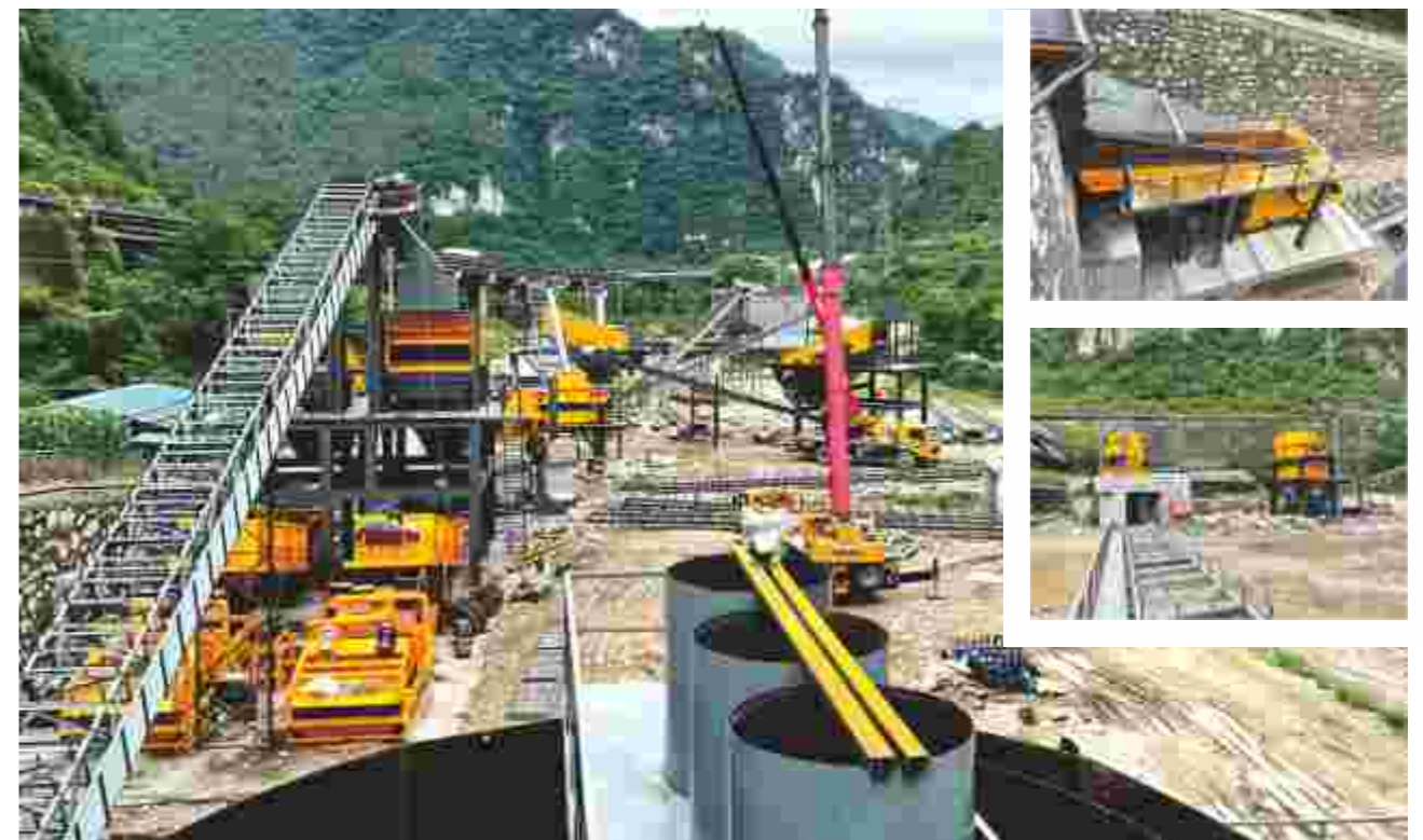
宜昌时产500~700吨鹅卵石原砂洗选及破碎整形生产线 Yichang 500~700 tons per hour of pebble raw sand washing and crushing line
